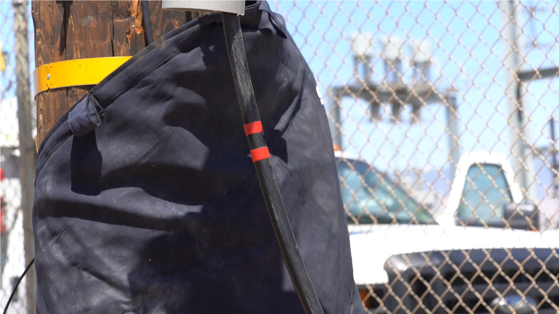
20 Second Fault initiates at 1.43, fault confirmation starts at 8.26
