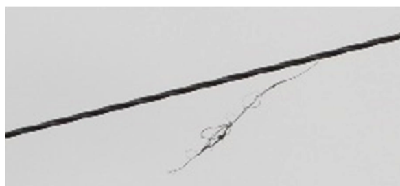
Figure 2: Cobweb on powerline detected by FireSafe SWER EFD system.
