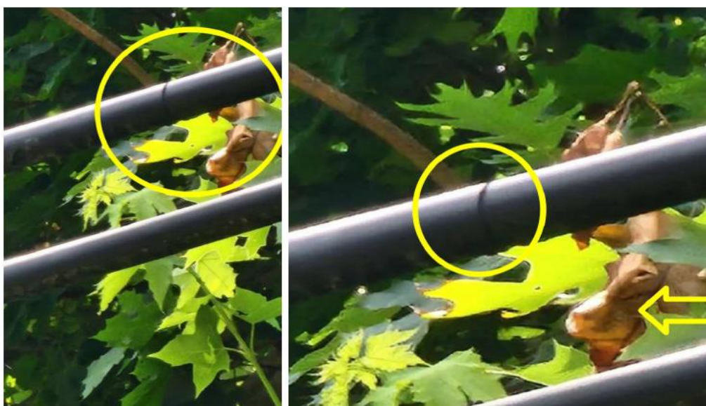
Figure 2: Cracked Spacer Cable
