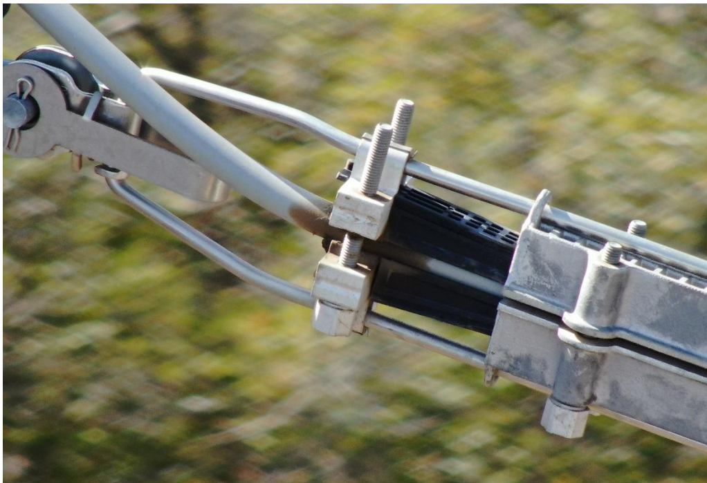
Partial discharge through compromised insulation discovered via Early Fault Detection (EFD)
