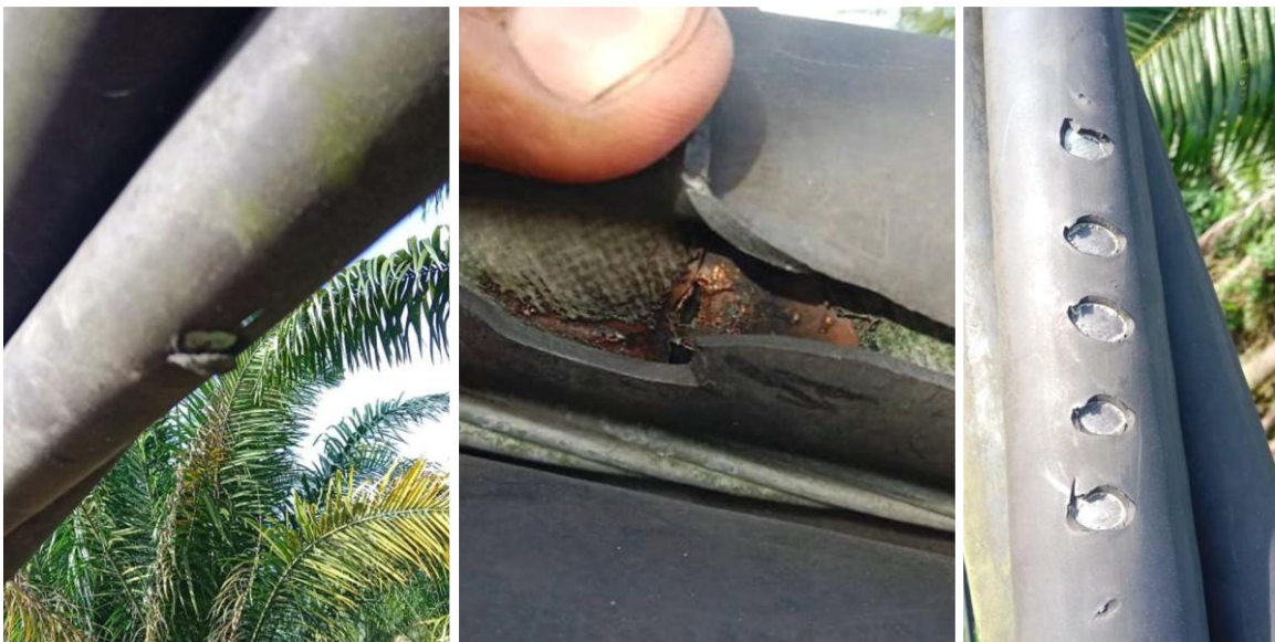
Insulation defects and compromise discovered via Early Fault Detection (EFD)
